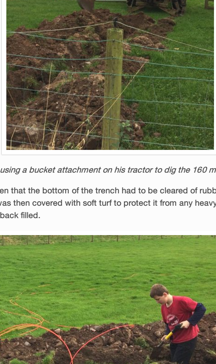
Steve Wilman using a bucket attachment on his tractor to dig the 160 metre long trench
