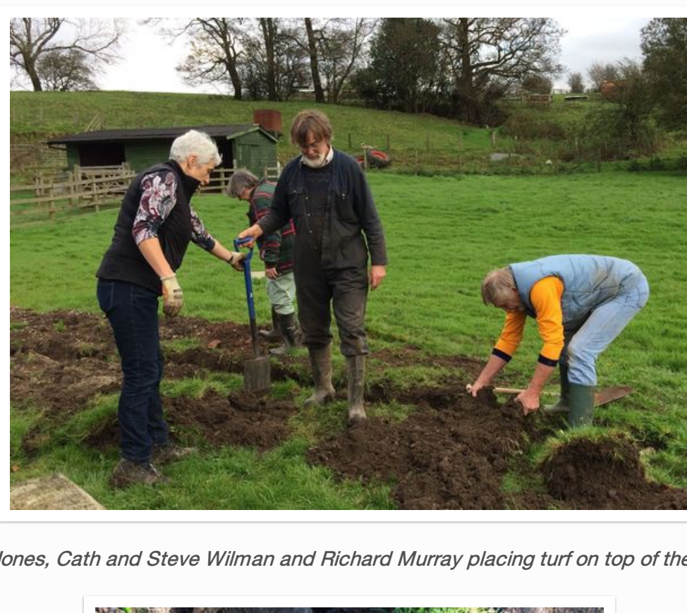
William Mawdsley, on half term holiday, smoothing the bottom of the trench before the ducting was laid
