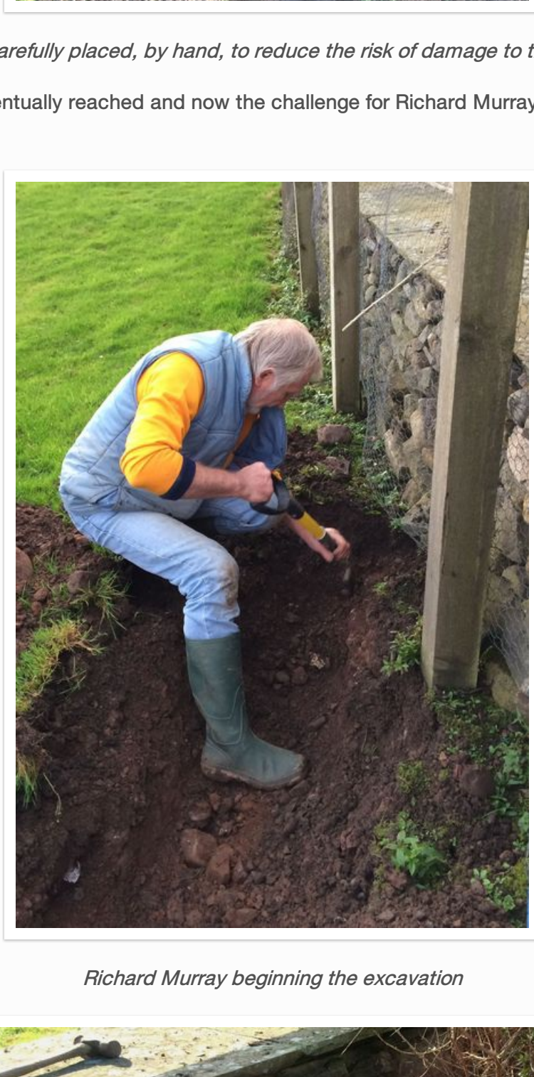
Stones carefully placed, by hand, to reduce the risk of damage to the ducting
